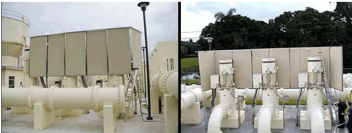
Figure 4.2 Acoustical Tiles on Pumps
